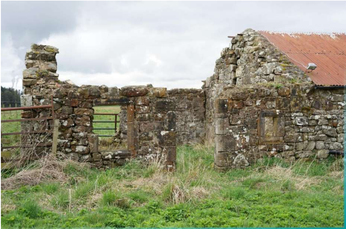
VP17a Southern section of Camilla: Building, illustrating loss of roof and general deterioration of condition
