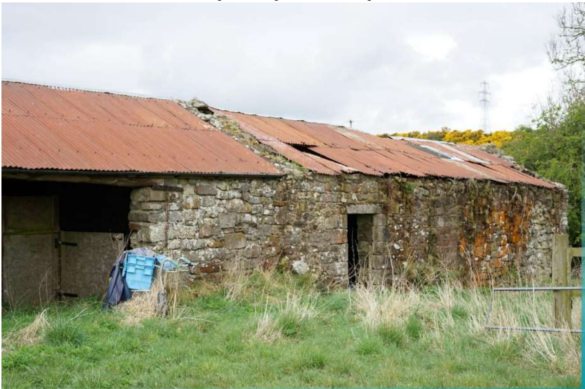
VP17b Northern section of Camilla: Building, showing general poor condition, in particular the corrugated iron roof
