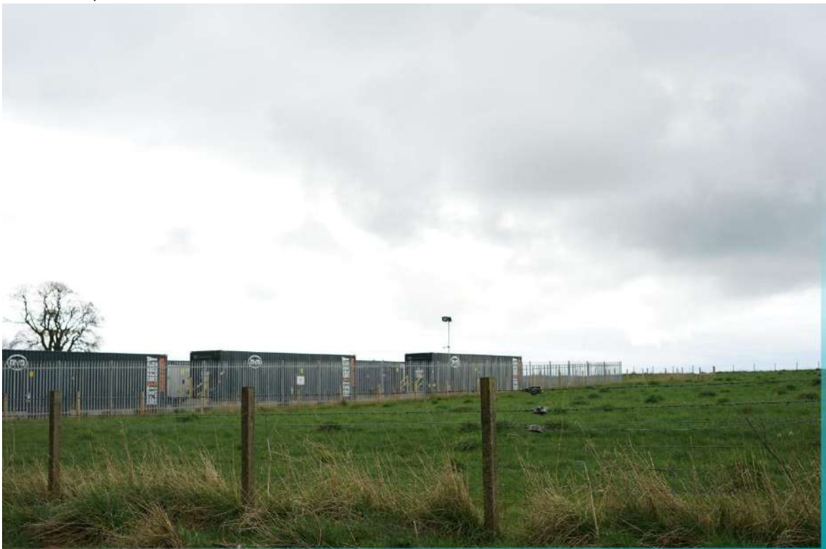
VP20 Camilla BESS looking east
